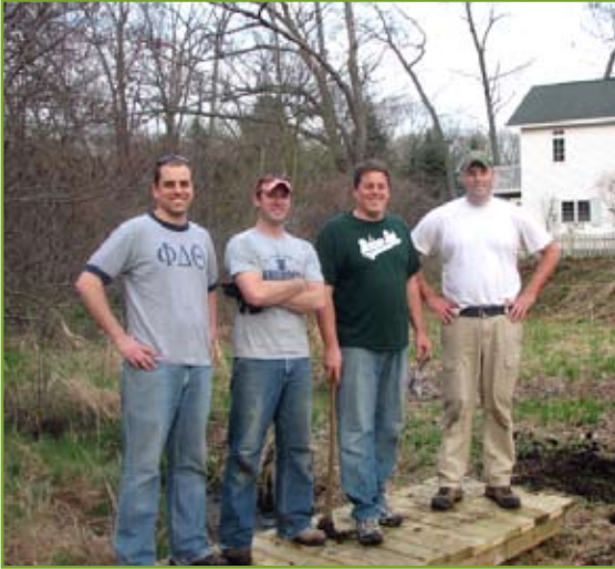
Stewardship volunteers constructed a bridge across the creek at the Minnie Skwarek Nature Preserve, connecting the hiking trail to the Grand River. Photo: Melanie Good
